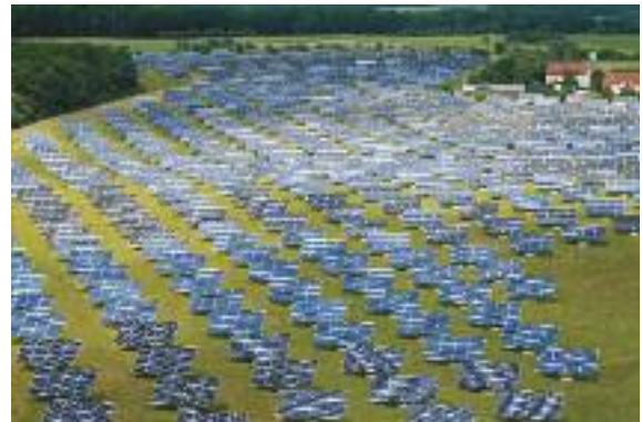
Large ground-mounted system in Germany.
