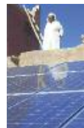
Off-grid PV system in Morocco.
