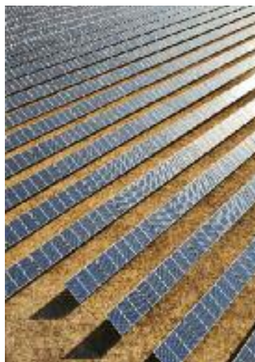
Large ground-mounted PV plant, Mallorca, Spain.
