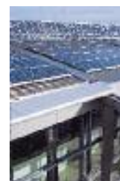
PV modules integrated into flat roof.
