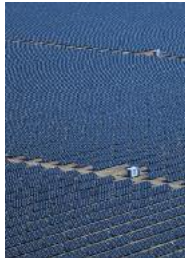
Large ground-mounted PV system in Spain.
